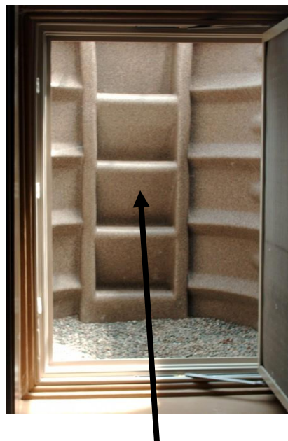
Looking from the basement through the egress window into the egress well.
